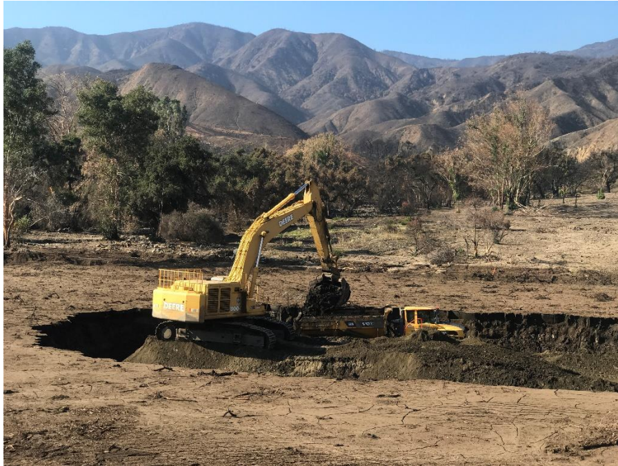
Figure 11.1: Leach Debris Basin Following 2018 Holy Fire
