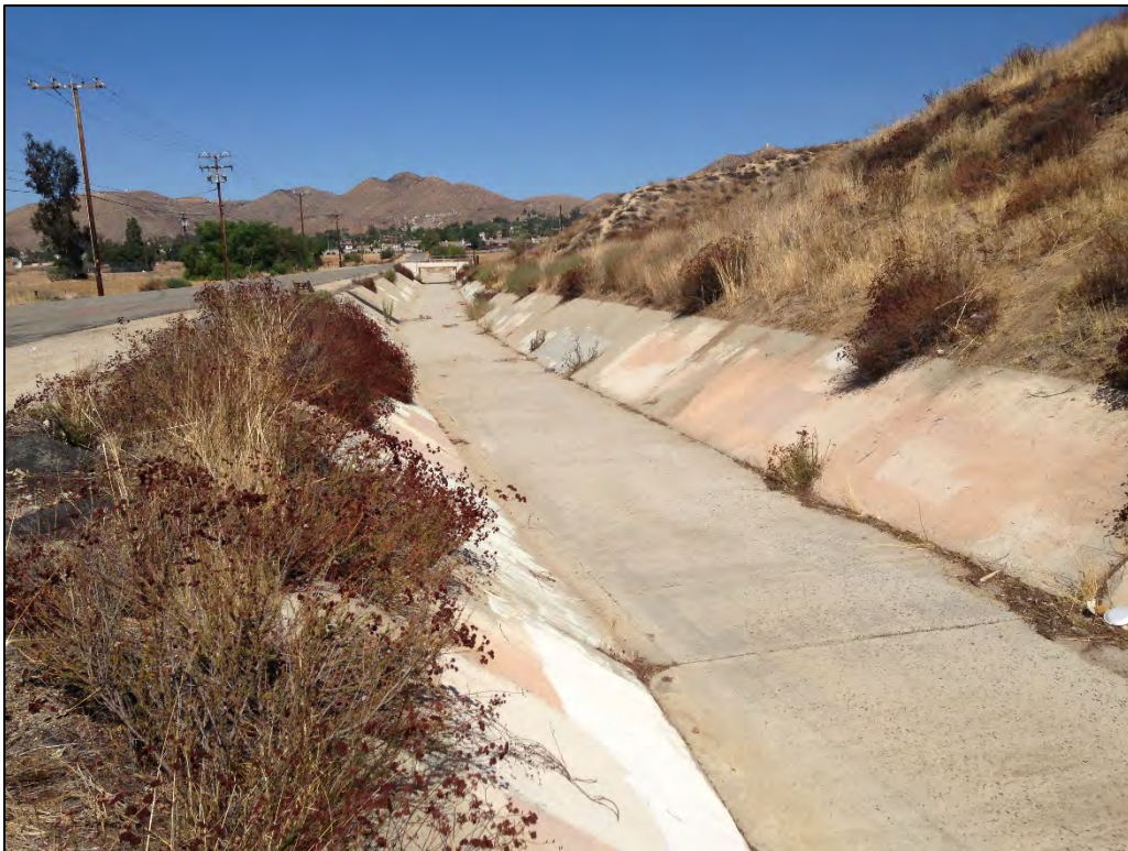
Photo 6. Existing concrete-lined drainage along Monte Vista Road, south of the proposed Bundy Canyon Basin; northern portion of proposed Lateral C Main Line
