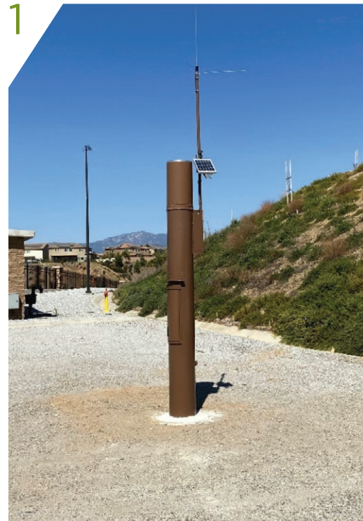
Real-time telemetered rain gauge installation (ALERT gauges): Calimesa at Singleton Road
